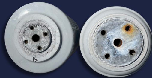
Thirteen insulators in one of the isophase ducts were damaged by water intrusion, which would have led to a forced outage.
